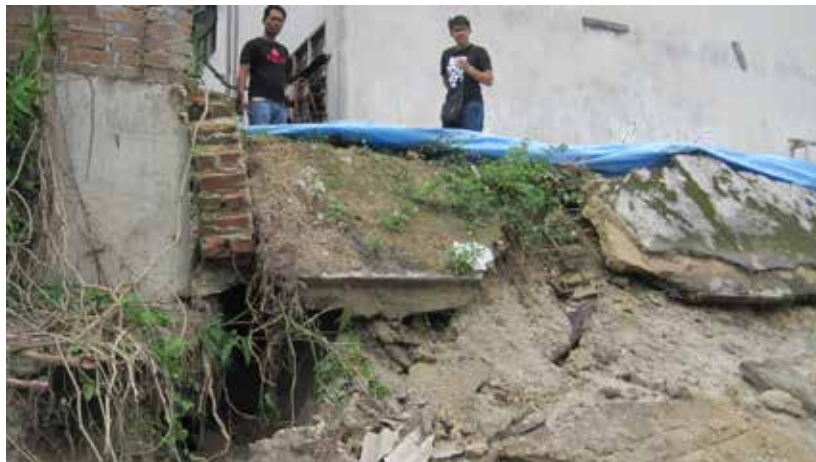
Lawatan lapangan berkaitan kejadian runtuh tembok di No.25F, Jalan Bunga, Kg. Tengku Hussein Lama, Manjoi, Ipoh. Field visit on the collapsed wall at No.25F, Jalan Bunga, Kg. Tengku Hussein Lama, Manjoi, Ipoh,
