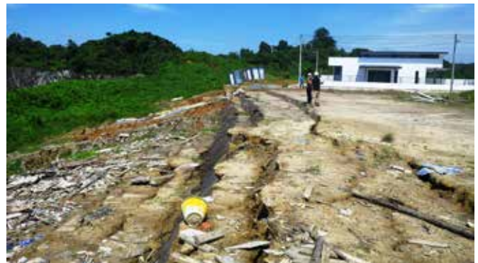
Siasatan tanah runtuh akibat peletupan batuan di Kuari CMS Sdn. Bhd., Kuching, Sarawak Investigation of blast-induced landslides at CMS Quarries Sdn. Bhd., Kuching, Sarawak
